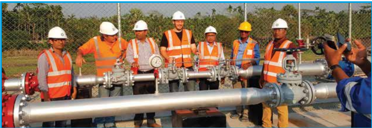
RMS Commissioning of M/S Aggreko Project International Limited (95 MW)
